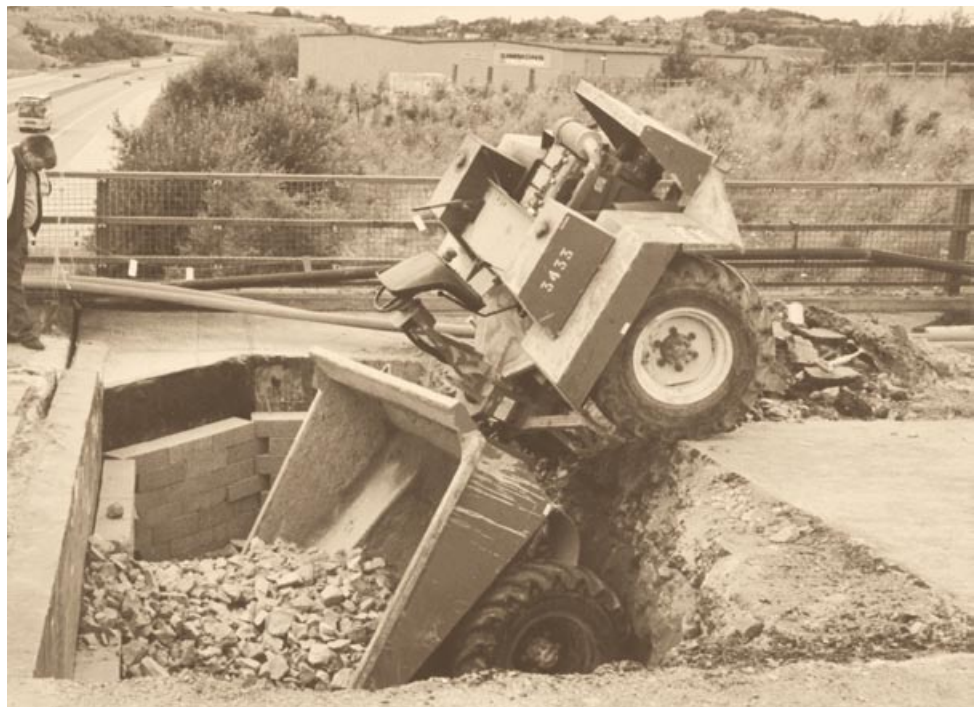
Figure 14 Small site dumper fallen into excavation due to lack of wheel stops
